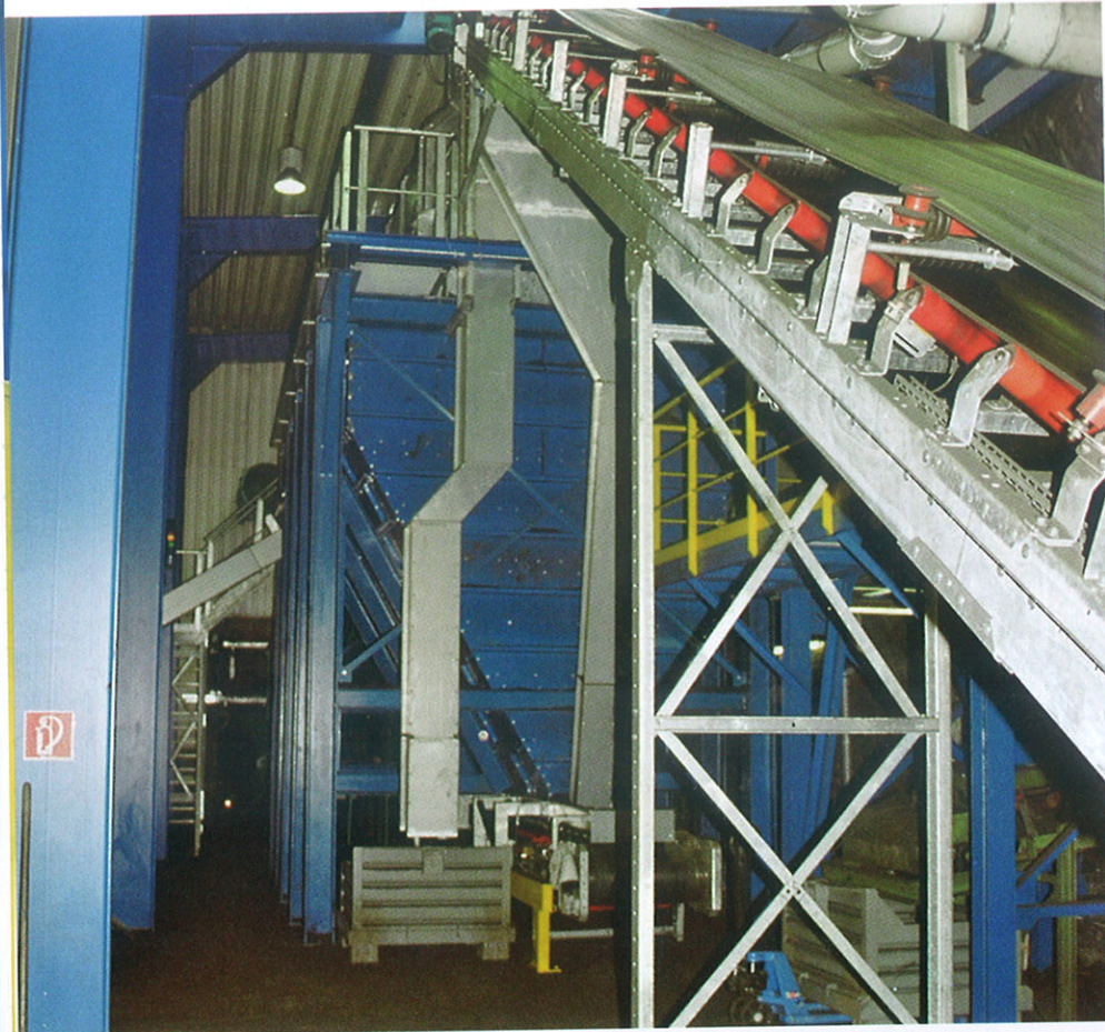
Figure 2: The new polygonal screen separates unusable sand clusters and sends them to the disposal area
